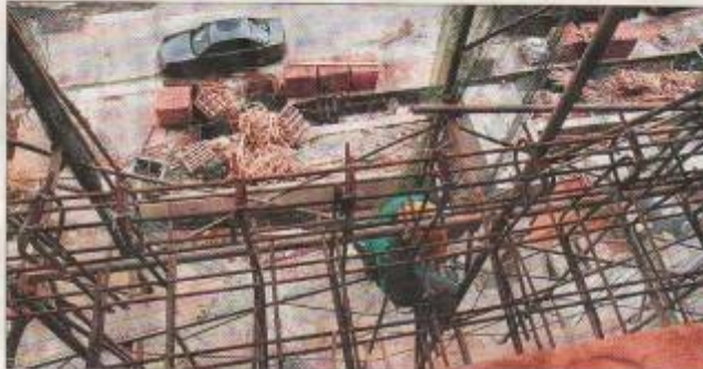
CARELESS: While poorly built scaffolds — such as those missing the guard rails required to keep workers from falling — are a key problem, there are also workers who do not attach their harnesses to the structures, a requirement for anyone working above a height of 3m.
